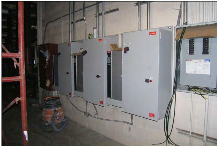
Architectural & Engineering Services- Electrical Panels
