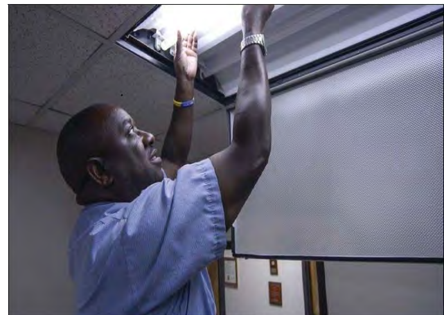
Building General Maintenance
